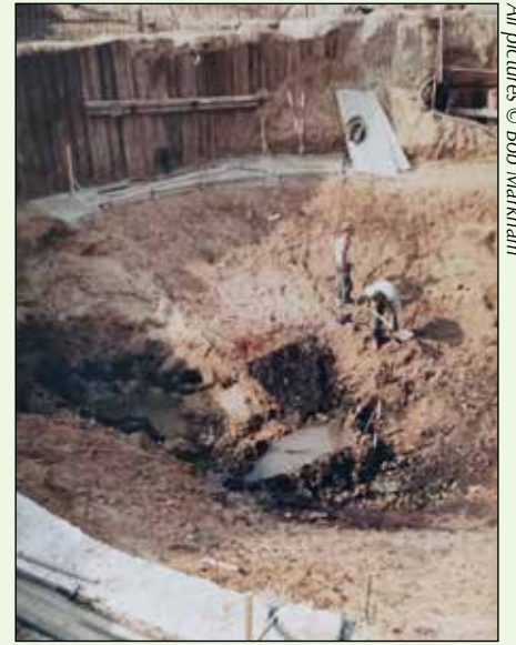
Sand and gravel rests on the black peaty deposits of the Ipswichian interglacial in the construction of extensions to the sewage works in 1967
