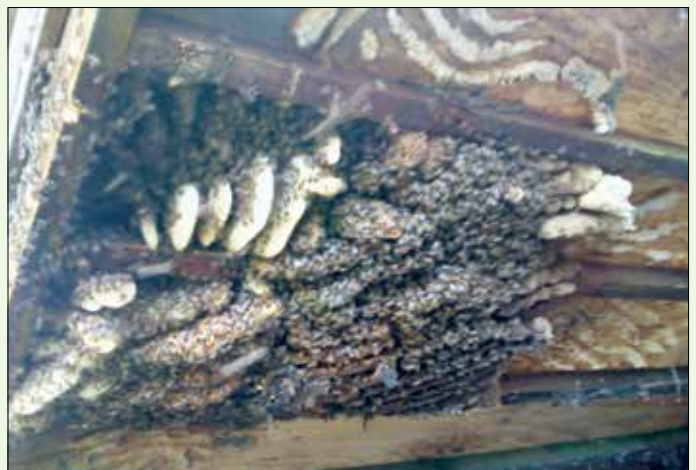
We had to carefully cut away the comb
