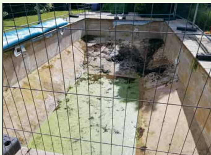
Pool slowly draining as liner has been removed. We sifted through the detritus with nets and trays
