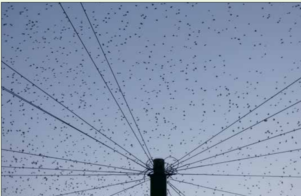
Poles and wires can be hazards to flying and perching birds
