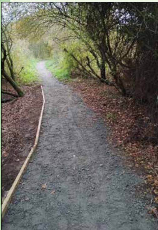
Part of the newly surfaced pathway from Bourne Park to Bobbitts Lane
